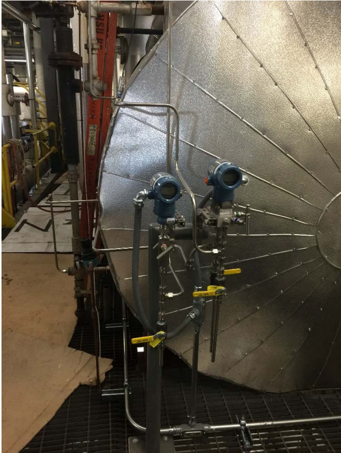
New Deaerator Tank Controls
