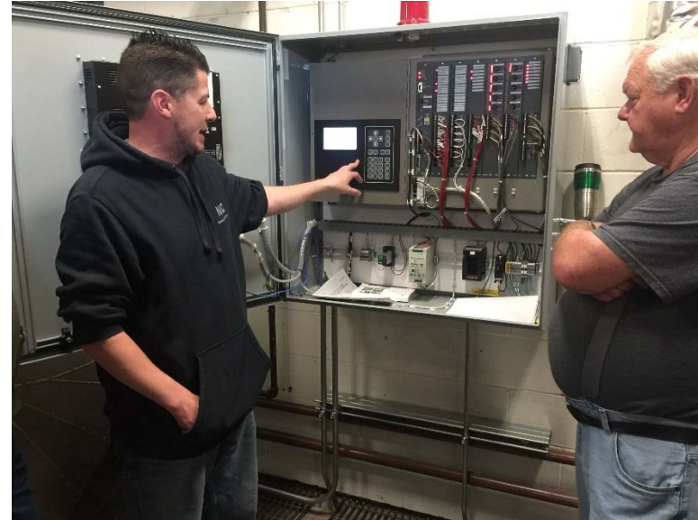
New Control Panel
